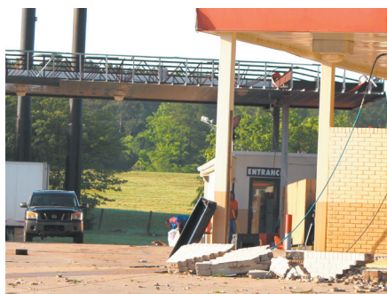
(Top) A light pole lands on a diesel truck behind the Chevron on Hwy. 43. (Bottom) The Texaco sustained damage to roof and structure walls. (Photos by Katie White)
